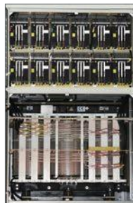
Power cell cabinet (Top) Transformer cabinet (bottom)
