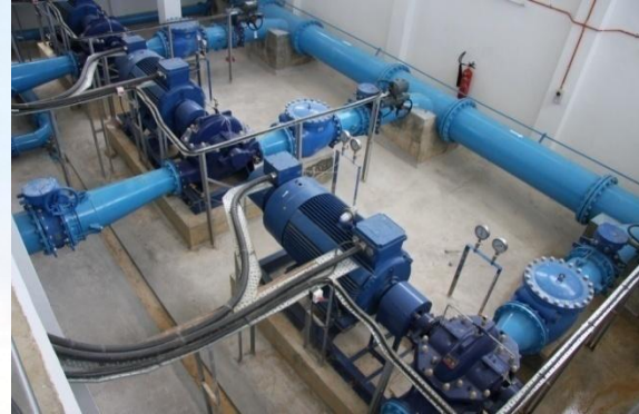
Water Plant, Malaysia
