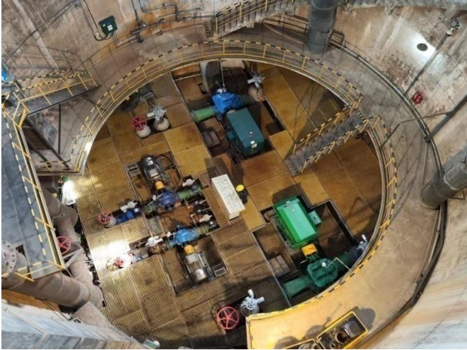
MAOTAI Factory water intake
