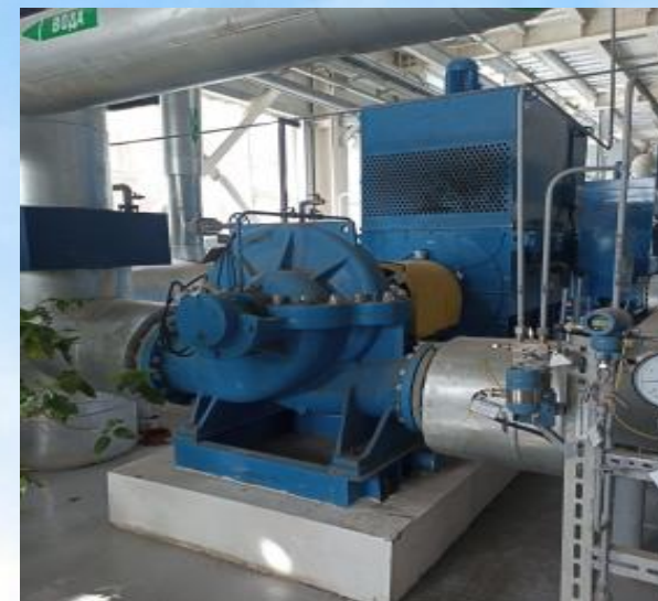
Boiler room, Izhevsk
