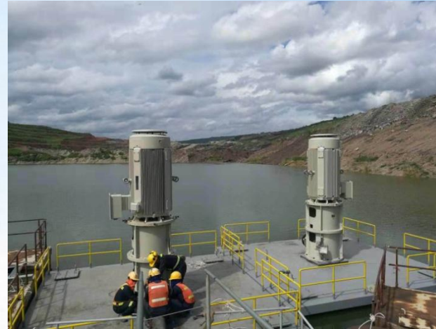
EGAT power plant ,Thailand
